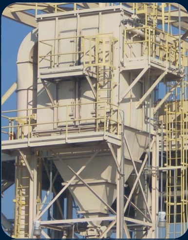
CPS Energy - Storage Bin
