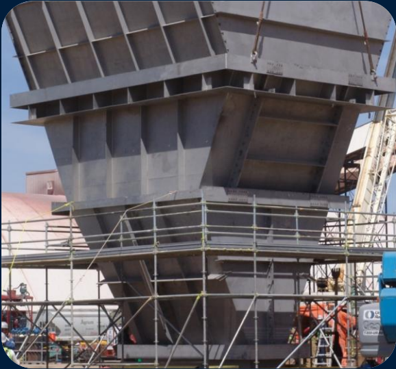
SNC-Lavalin Inc.: Saskatchewan, Canada Fine Ore Storage Bin – 2205 Stainless Material (1 of 3 Total Bins Supplied)
